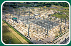
BALSIK EXTRA HIGH VOLTAGE SUBSTATION COMPLETED: APR 2022
