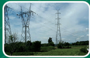
SAN ESTEBAN-LAOAG 230KV T/L COMPLETED: FEB 2017 COST: PhP3.24 BILLION
