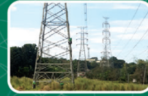
SAN JOSE-QUEZON 230KV LINE 3 COMPLETED: NOV 2020 COST: PhP1.55 BILLION
