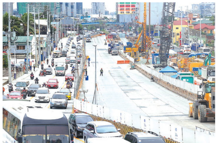
PHILIPPINE STAR/MIGUEL DE GUZMAN THE CONSTRUCTION of the Metro Manila Subway Project-Tandang Sora station is seen in this file photo taken on Jan. 12, 2025.
