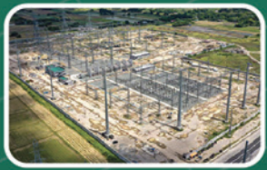
BALSIK EXTRA HIGH VOLTAGE SUBSTATION COMPLETED: APR 2022
