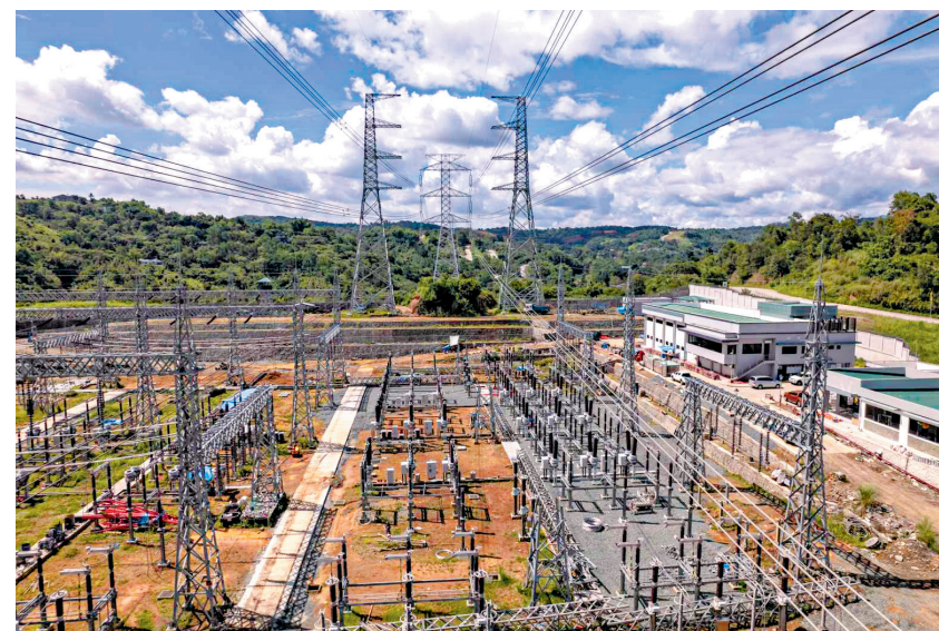
UNPARALLELED EXPERTISE. MIESCOR has consistently been recognized by the Philippine Contractors Accreditation Board (PCAB) with a Quadruple A or "AAAA", the highest license category for engineering, building and specialty electrical mechanical and communication facilities contractor, since 2018.
