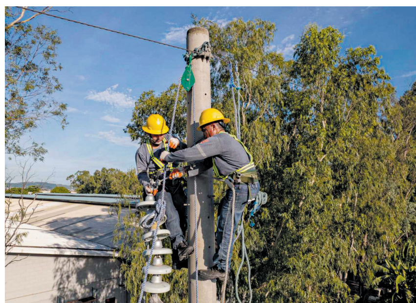
THE FORCE BEHIND POWER. MIESCOR provides various services to distribution utility companies including Meralco, the country's largest distribution utility company.
