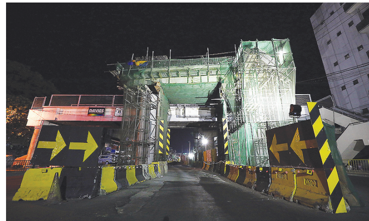
A CONSTRUCTION SITE is seen along Quirino Avenue, Manila in this April 3, 2020 file photo.
