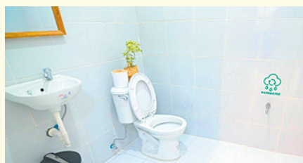
Faucets connected to the rainwater catchment are duly marked to help guide the community.
