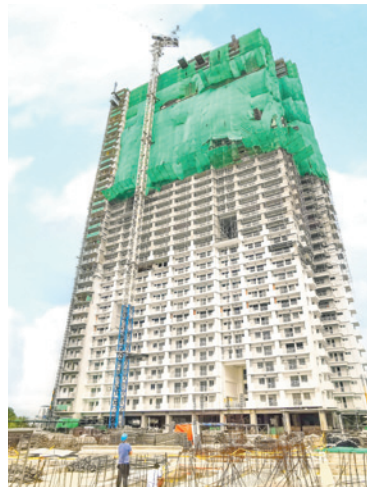
THE 40-storey building called Cadence is set to be turned over on June 24.
