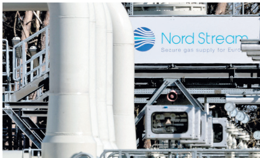
PIPES at the landfall facilities of the Nord Stream 1 gas pipeline in Lubmin, Germany.
