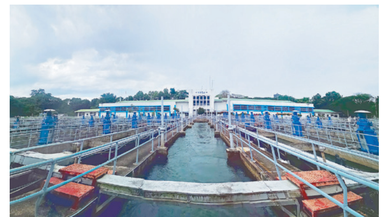
Balara Treatment Plant 2
