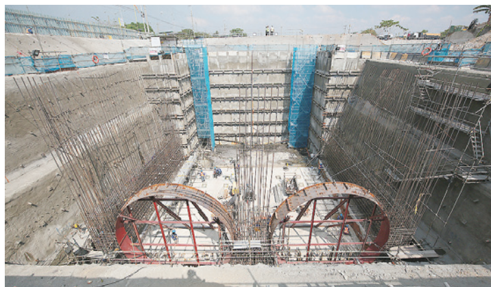
CONSTRUCTION of the Metro Manila subway project is seen in Valenzuela, March 8.
