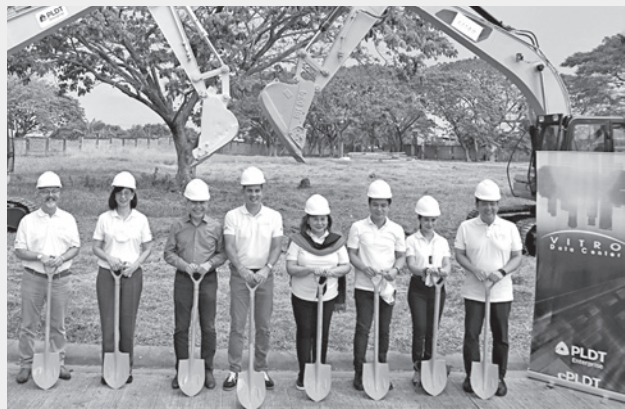
MERALCO TO POWER PLDT'S 11 TH AND LARGEST VITRO HYPERSCALE DATA CENTER LOCATED IN STA. ROSA, LAGUNA. Present during the groundbreaking ceremony last March 18 were (from L-R): RED Engineering Regional Director for Asia-Pacific Martin Webb, DICT Regional Director Cheryl C. Ortega, Meralco President and CEO Atty. Ray C. Espinosa, PLDT and Smart President and CEO Alfredo S. Panlilio, PEZA Director General Charito B. Plaza, Laguna Governor Ramil L. Hernandez, Sta. Rosa City Mayor Arlene B. Arcillas, and PLDT FVP and Head of Digital Office Viboy S. Genuino. (Photo courtesy of PLDT)
