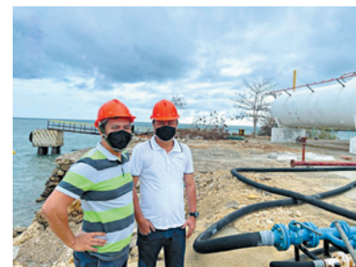
Employees in Brgy. Langtad, Naga City, Cebu conducted plant inspections to ensure sufficient LPG supply in the area.
